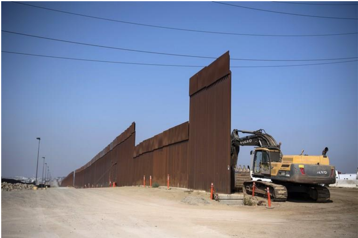
Construction is seen on the secondary fence that separates the United States and Mexico in the San Diego Sector on Aug. 22, 2019 in San Diego, Calif.
